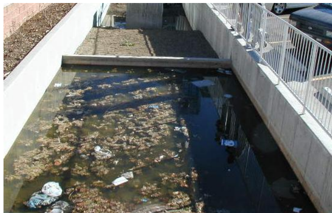
EXHIBIT 1.4 STORMWATER BMPs SHOULD BE DESIGNED AND MAINTAINED TO PROTECT PUBLIC HEALTH AND AVOID NUISANCE CONDITIONS
