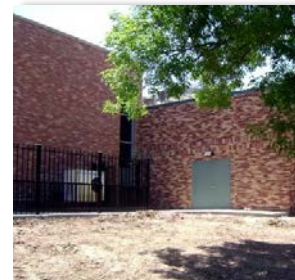
New Coolerado cooling units
