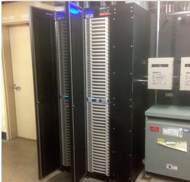
New lighting controls
