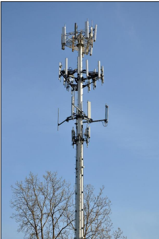
Typical large cellular antenna.
