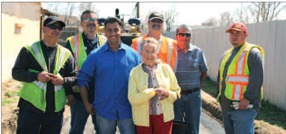
Longtime residents Fern Veasman (center) and Robert Duran (second from right) along with Councilman López thank alley paving work crews.
