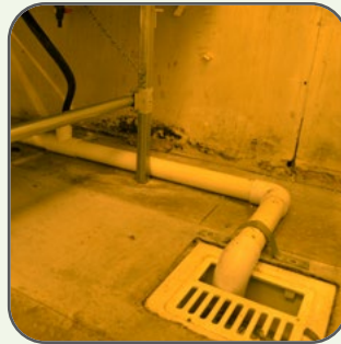
Figure 7: Piped drainage running into floor sink
