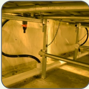
Figure 6: Example of piped drainage from trays
