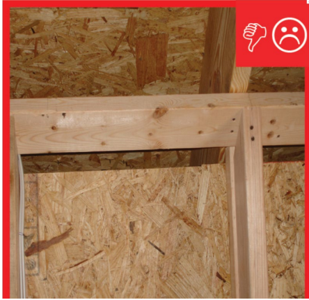
Air barrier not continuous
