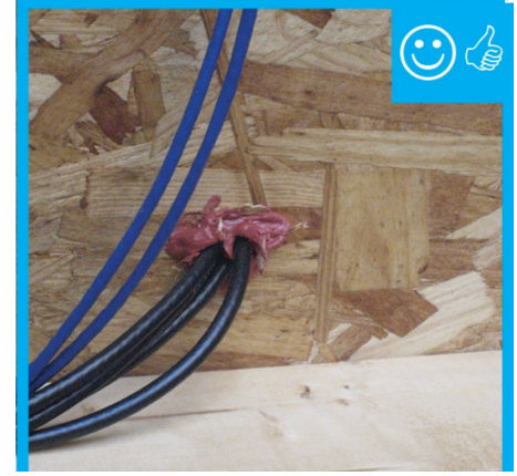
Wiring penetrations nicely sealed
