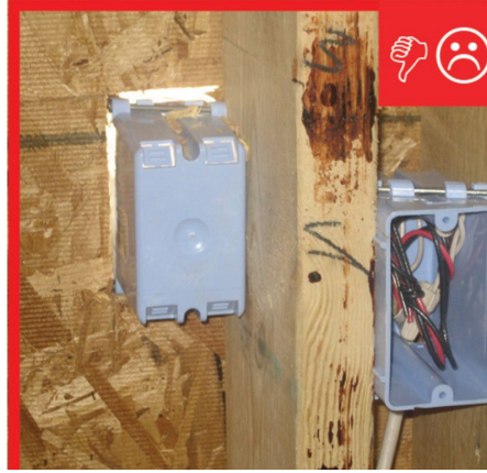
Electrical box not sealed
