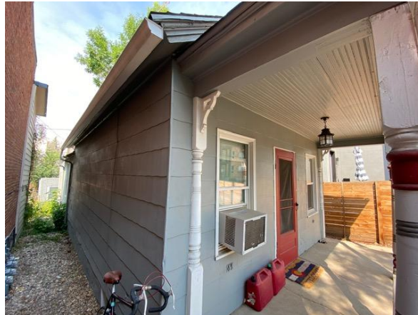
EXISTING FRONT OF HOUSE WITH EXISTING NON-HISTORIC ALUMINUM WINDOWS (LEFT)
