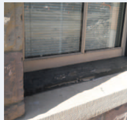
Top Right: Repair work underway to damaged and deteriorated features. Middle Right: A damaged limestone sill. Bottom Right: The repaired limestone.
