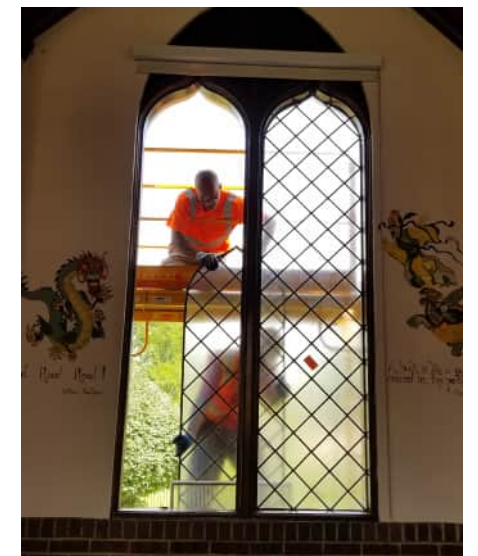
Top: Molly Brown House after exterior restoration. Middle: Denver Dry Goods undergoing restoration Bottom: Window restoration and re-installation at Denver Academy.
