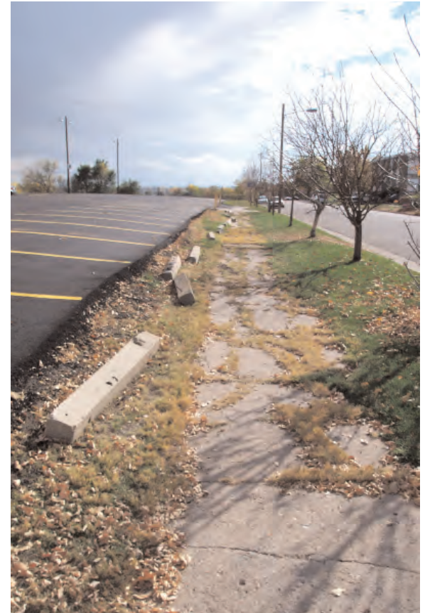
Aging pedestrian infrastructure creates an uncomfortable walking environment and conveys an image of neglect that threatens neighborhood stability.
